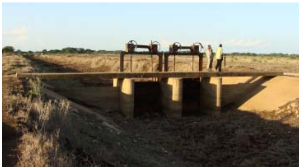
Sluice in TDIP Main Canal. This picture was taken at the height of Block B, South of Kulesa.
